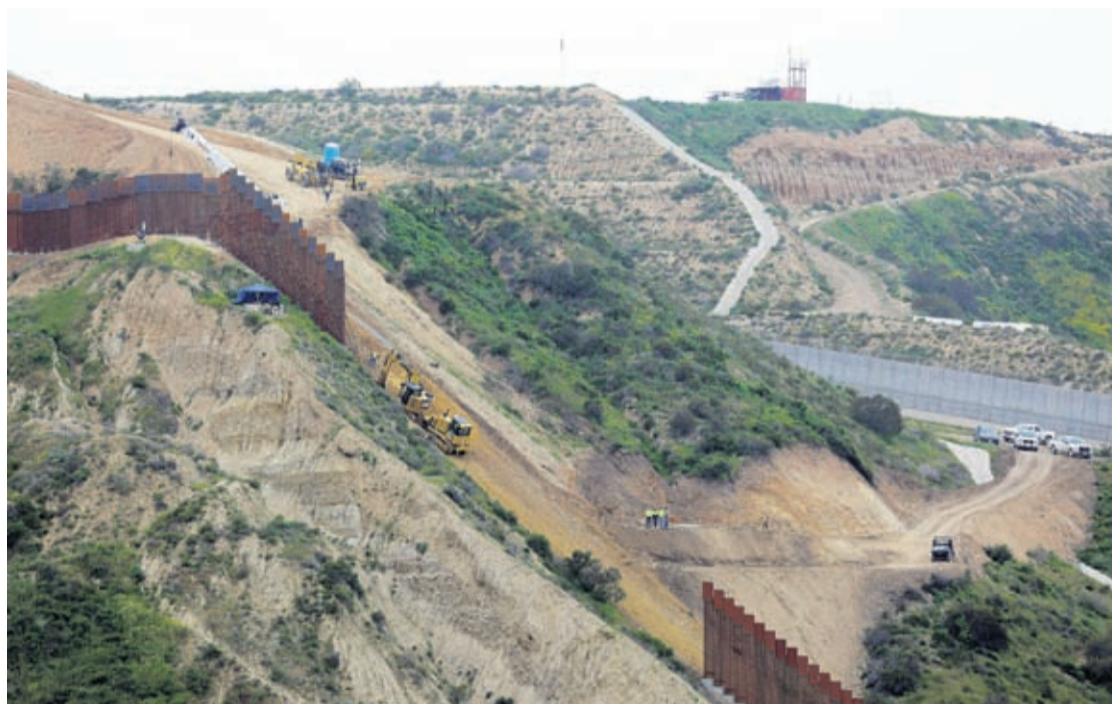
In this March 11, 2019 photo, construction crews replace a section of the primary wall separating San Diego, above right, and Tijuana, Mexico, below left, seen from Tijuana, Mexico.
